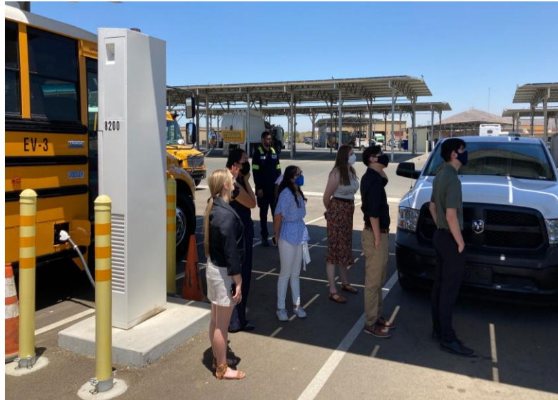
Figure 50: Student interns learning about EV charging at the City of Porterville bus yard.
