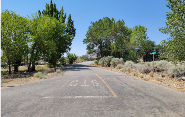
Missing sidewalks and bike facilities along School Street
