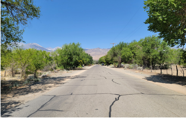
Missing sidewalks and bike facilities along Blake Street
